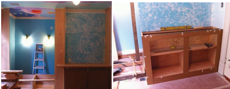
Figure 7: Building carcass for alcove drawers, futon mattress and the cabinet; mocking up cabinet face frame.
