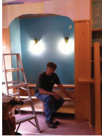
Figure 8: Mocking up the shape of the main archway; choosing wood for “legs” and main arch.
